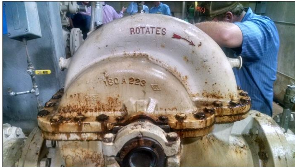
Raw Water Pump #2
