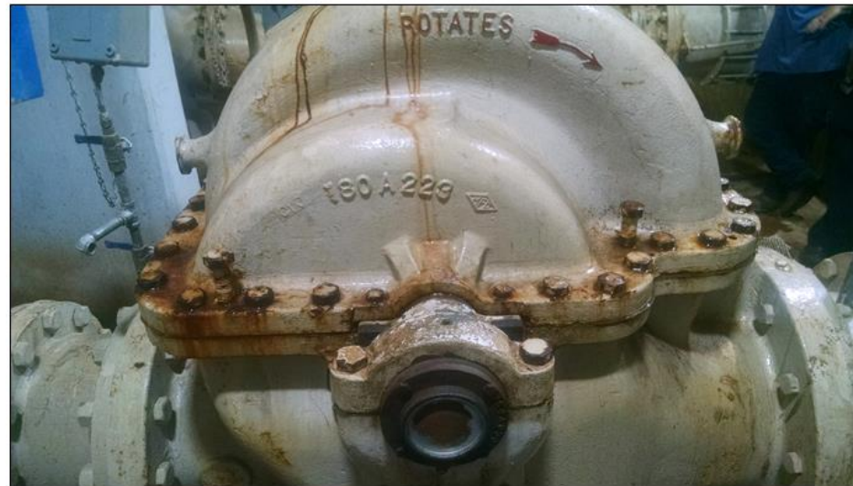
Raw Water Pump #1
