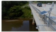
Flood Warning System
