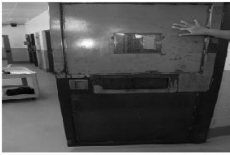
Door needs replacing
