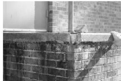
Back loading deck – Needs repairing
