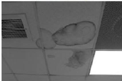
Damage from condensation from HVAC System
