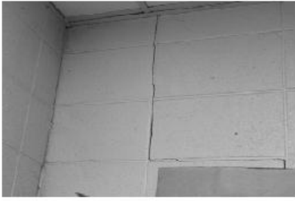
Cracks in the Block Walls
