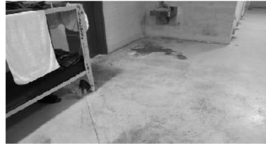
Floor needs painting
