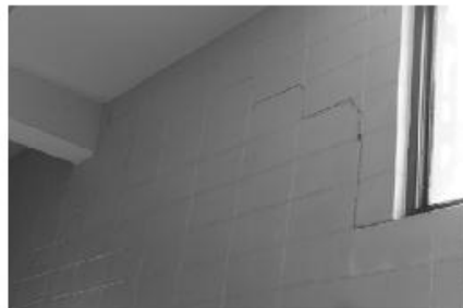
Cracks in the Walls – Female Dorm
