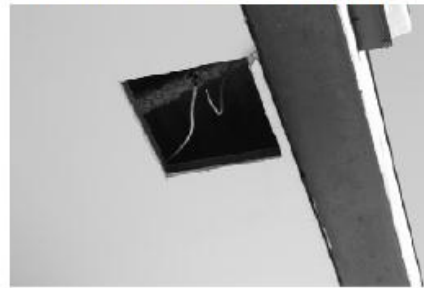
Open hole allowing birds to small area in roof due to Eve Dropping issue
