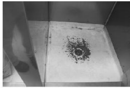
Floor in Shower stalls need painting
