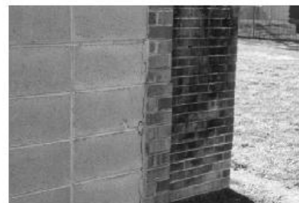
Maintenance Issues – Cracks, Moss
