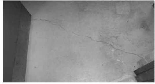
Cracks in the Block Walls
