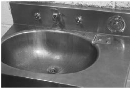
Sink for inmates – Water leaks
