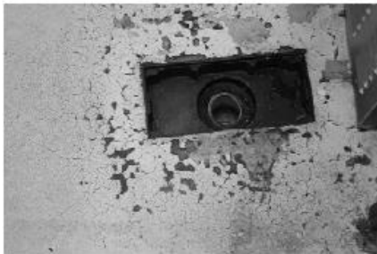
Drain area in Kitchen needs painting
