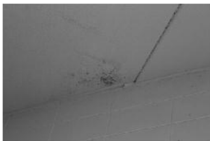
Water Damage from roof leaks
