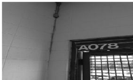
Cracks in the Block Walls
