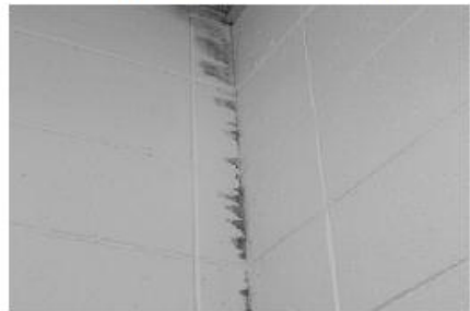
Water leak in adjoining outside wall – wind blown water leak
