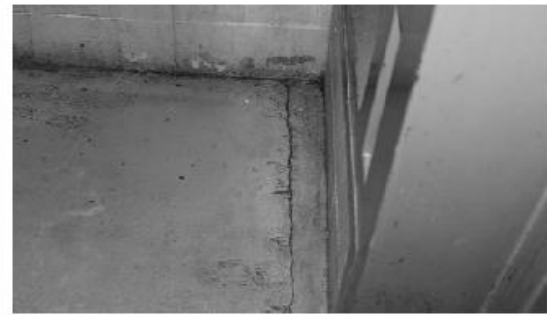
Maintenance Issues Crack in Floor
