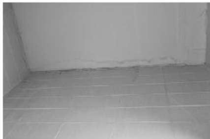
Water damage from water leaks
