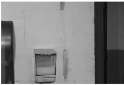
Attempted repair in wall crack.
