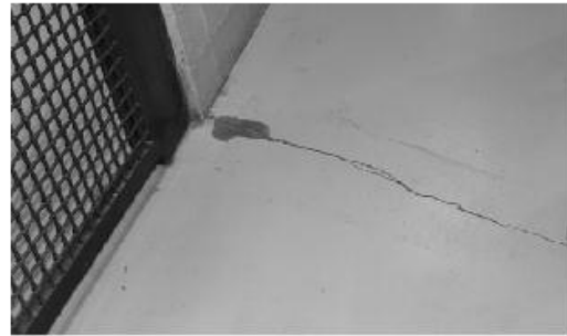
Cracks in the Floor - repair and paint
