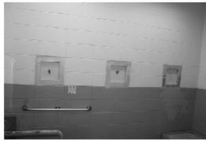
Medical Isolation Cell – Not a true isolation system – no separate air system
