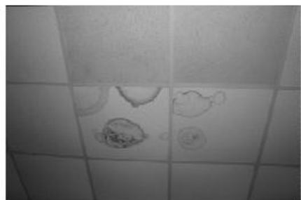
Damage from HVAC Condensation
