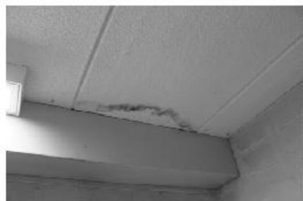
Water Damage - Roof leaks C and D Dorms
