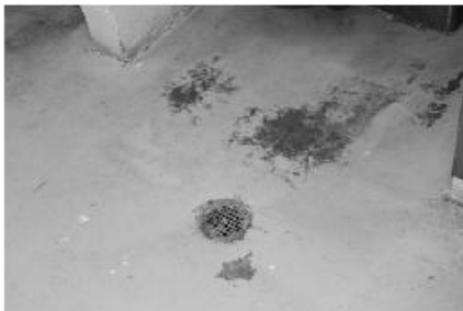
Floors need painting
