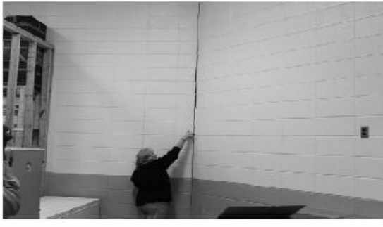
Separation of Exterior walls
