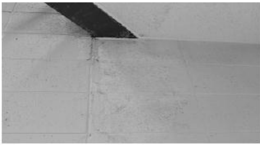
Water damage to wall from Roof Leak
