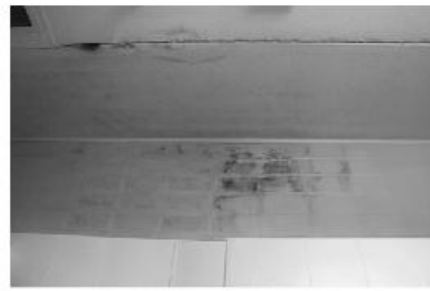
Major Damage from roof leaks
