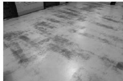
Floor Needs Painting
