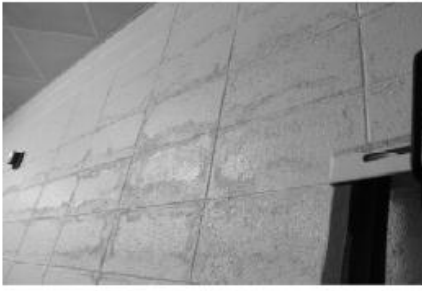
Wall damaged due to water damage
