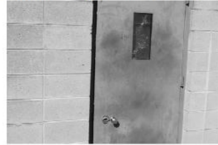
Door Lock system needs replacing – Current security system is obsolete
