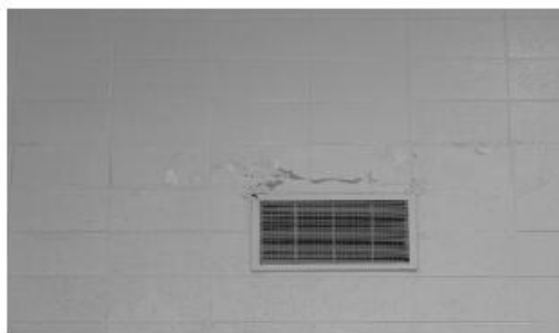
Attempted repair to a crack.
