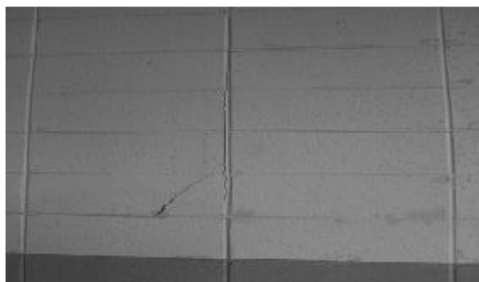
Cracks in the Block Walls
