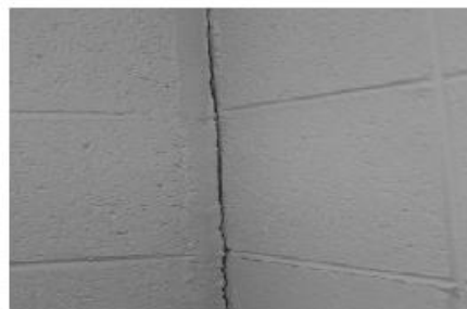
Cracks in the Kitchen Walls
