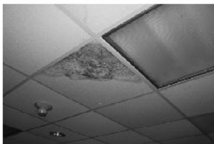
Tile Damage from Condensation- HVAC
