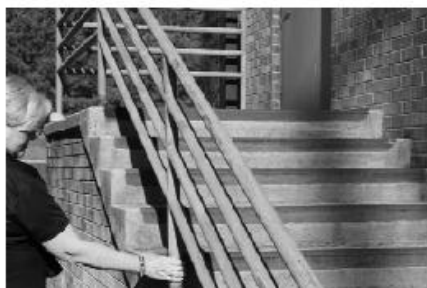
Maint. Issues – Rails need painting
