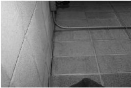
Water leak and crack in Laundry room
