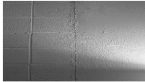
Seam needs to be repaired
