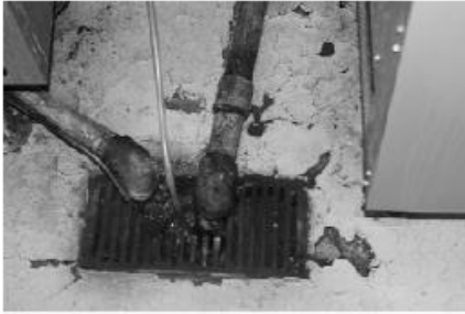
Kitchen Steamer drain area/system needs immediate attention
