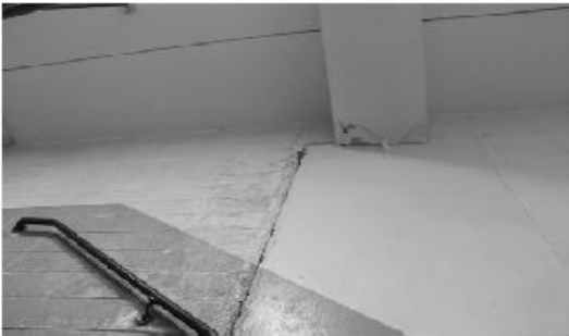
Damage from water leaks
