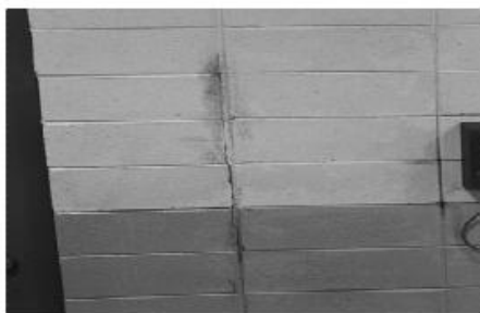
Cracks in Walls in Female Dorm
