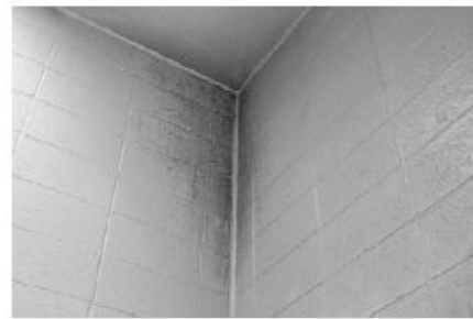
Residue from roof leaks
