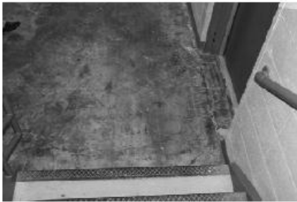
Floor tile needs to be replaced.
