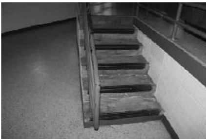
Maintenance - Tile needs replacing
