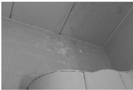
Damage from roof leaks
