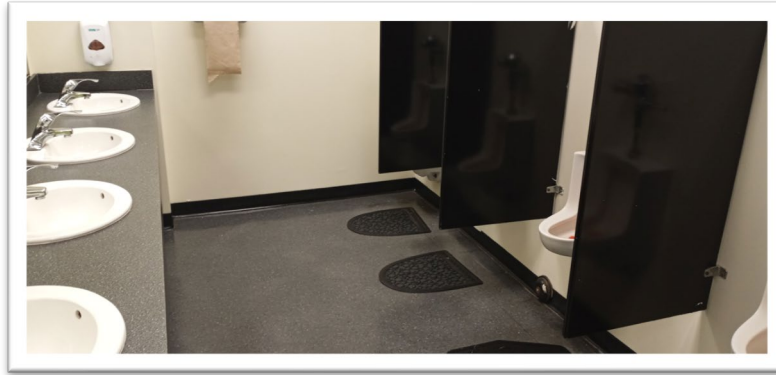
Figure 38: Main Lobby Men's Bathroom Clearance
