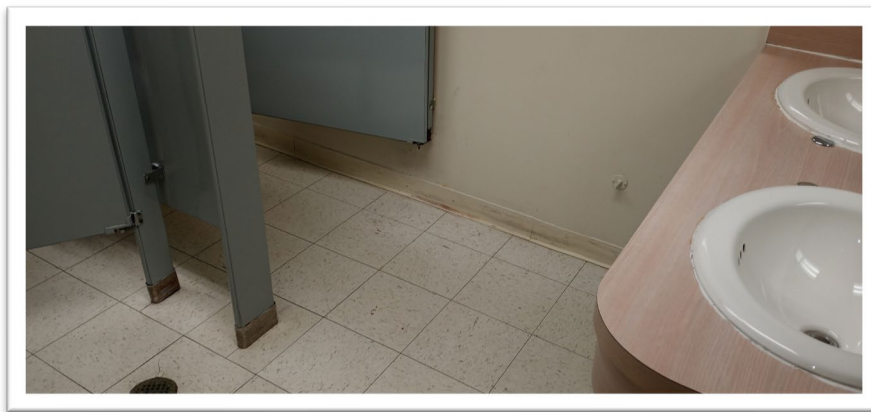
Figure 59: Senior Center Women's Lobby Bathroom Clearance
