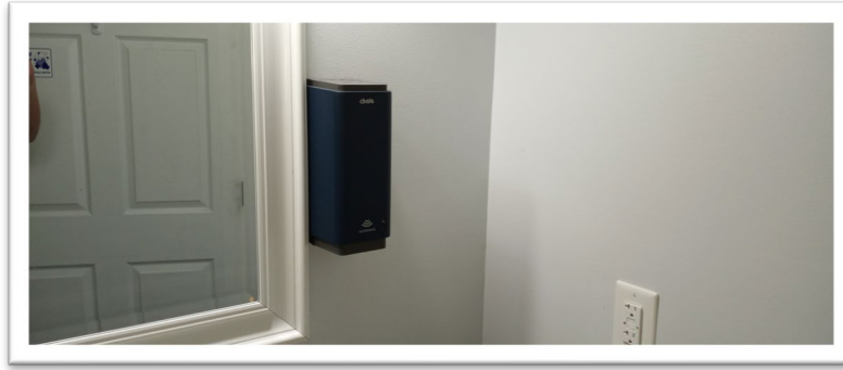
Figure 84: Public Works Single User Toilet Room Soap Dispenser
