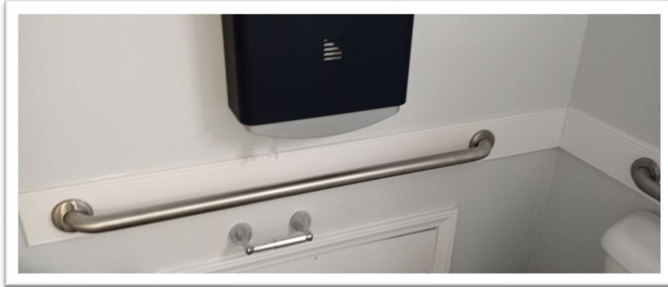
Figure 87: Public Works Single User Toilet Room Side Grab Bar
