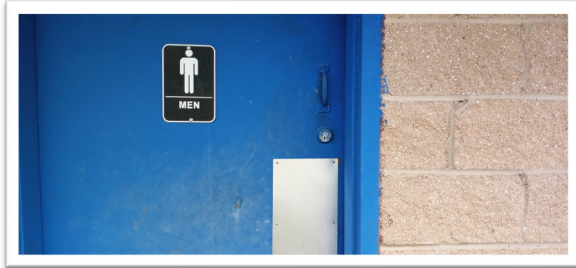
Figure 28: Men’s Bathroom Lock and Signage
